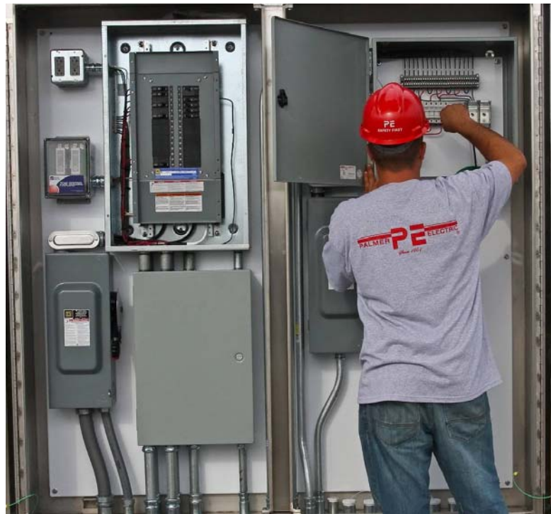
AC Side of Cabinet
